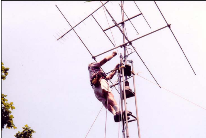
Jack, KA3ZLR, (Top) and Jack, K3DMY (above) work to erect antennas and towers.
